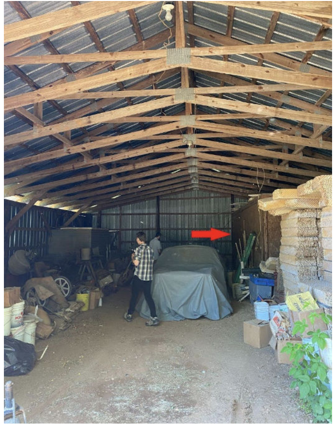
Figure 2. Large storage shed with internal room for conversion to mushroom fruiting location (red arrow).
