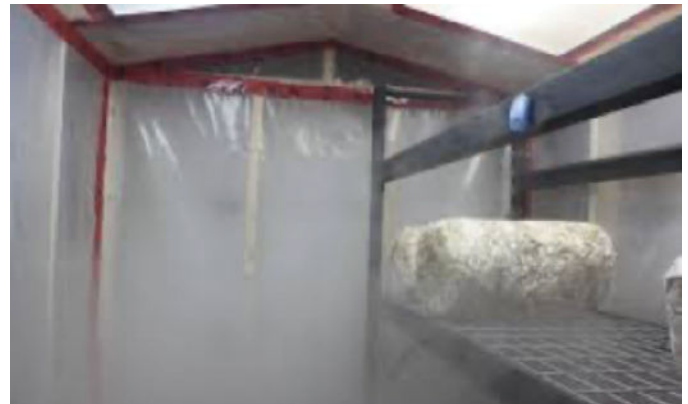
High Humidity in Room
