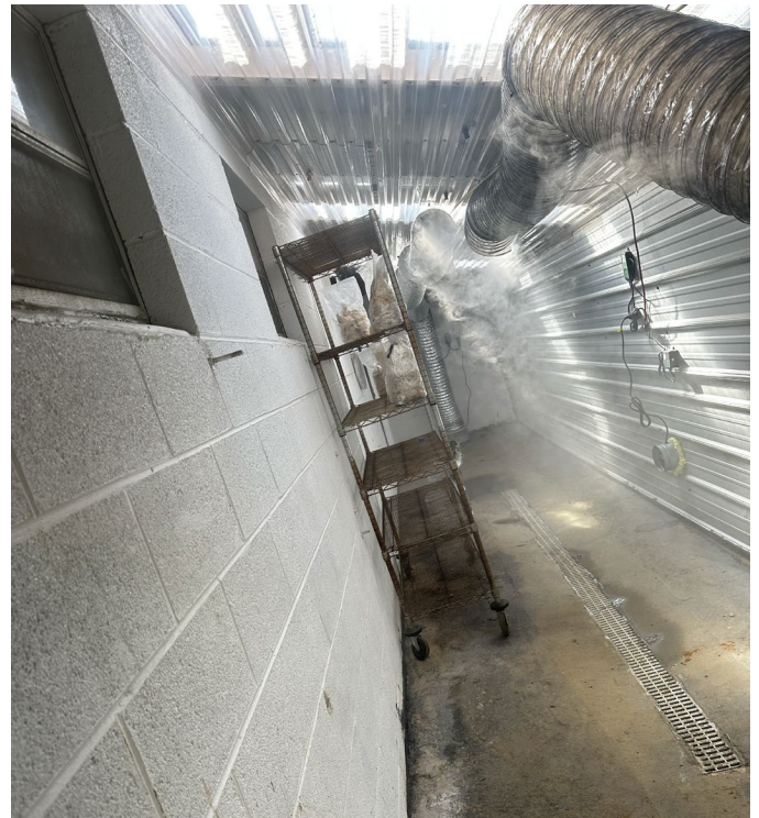
Mushroom-growing room with drains and environmental controls
